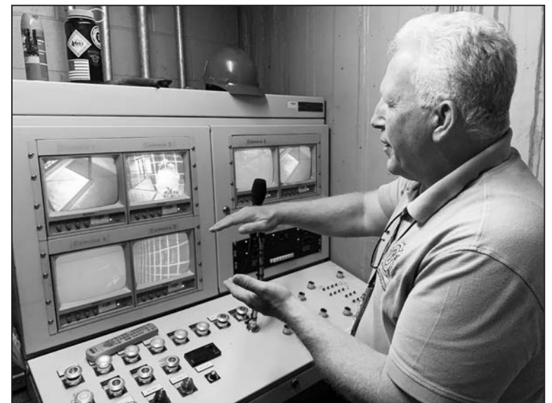
The new SCBA Maze Trailer replaces a 40-year-old permanent installation with obsolete electronics, seen here, that has exceeded its useful lifespan.
