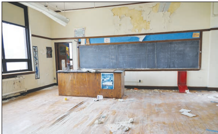
A classroom sits empty as years of deterioration are visible throughout the space.
