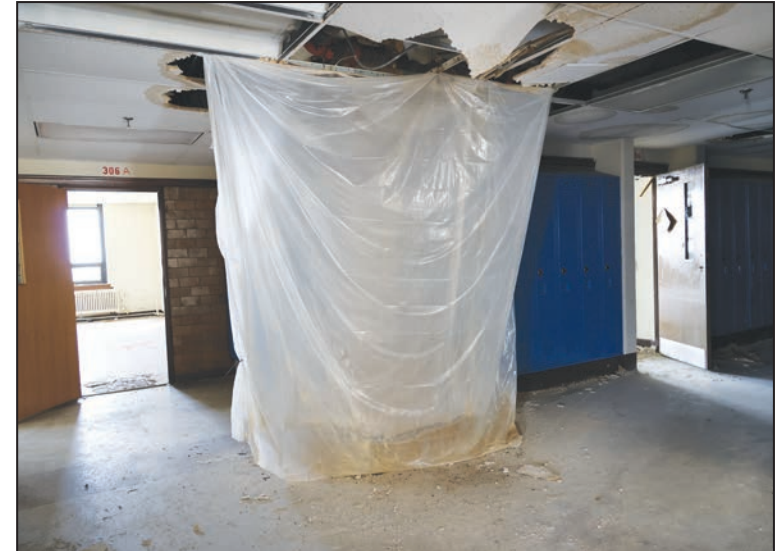
A tarp hangs from the ceiling where there are signs of water damage.
