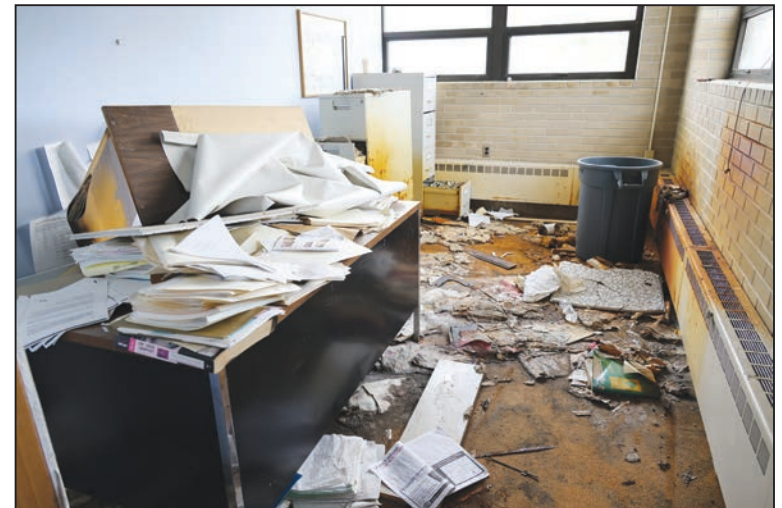
Years of vacancy have left this room covered in debris, illustrating the extent of deterioration in previously unused areas of the building.
